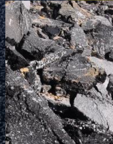
Broken Asphalt Pavement
